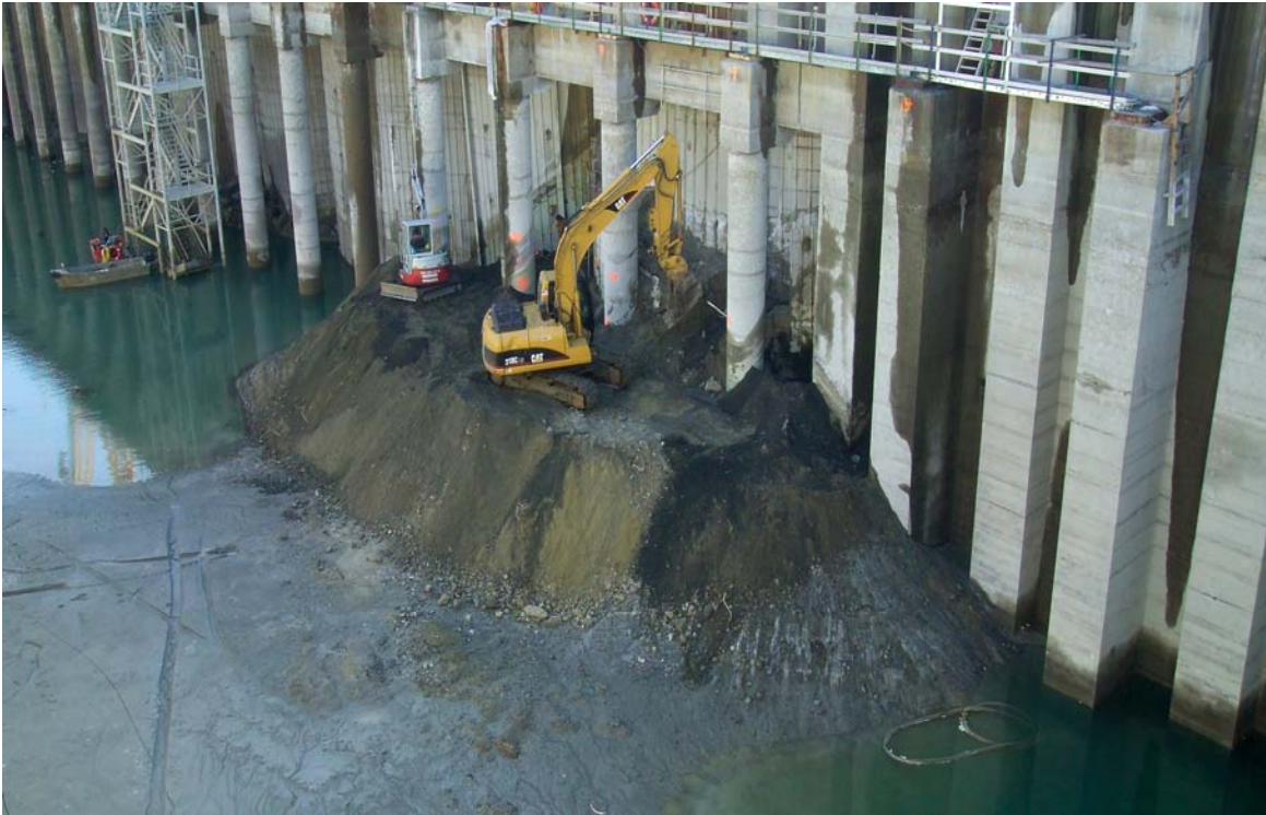
Figure 3 – Inboard side of GD-3 Cell S-2 showing backfill from ruptured interlock
