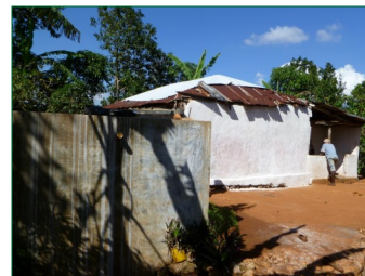
One of 93 houses needing roof repairs.
