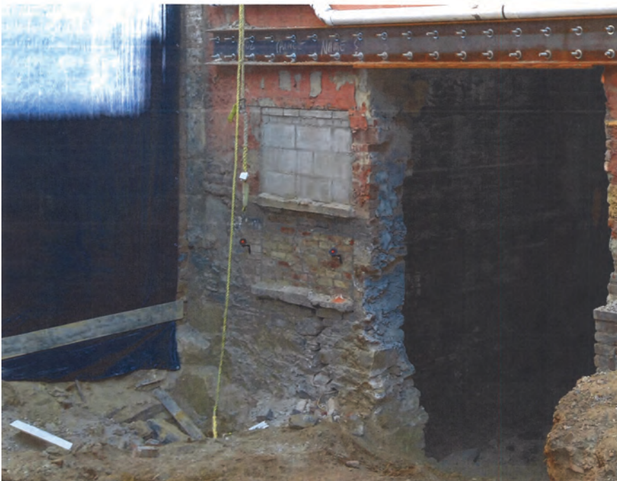
Figure 2. Prisms monitoring large crack in a building.
