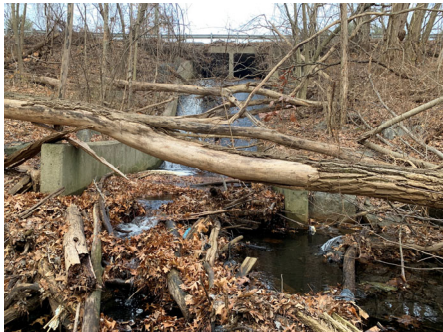
Spillway chute with fallen trees that needs replacement
